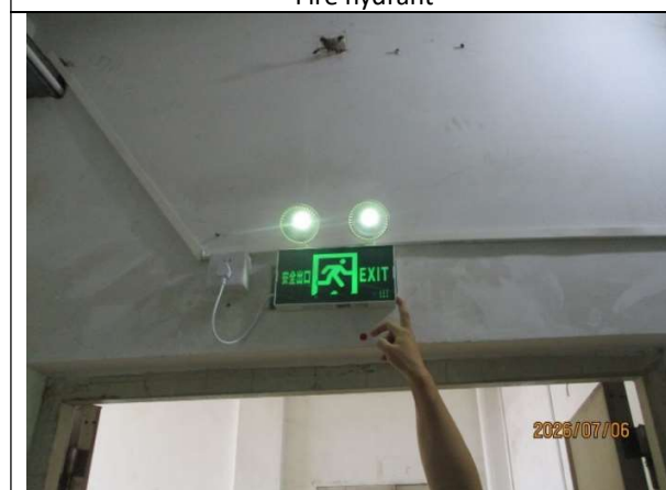
Emergency light testing
